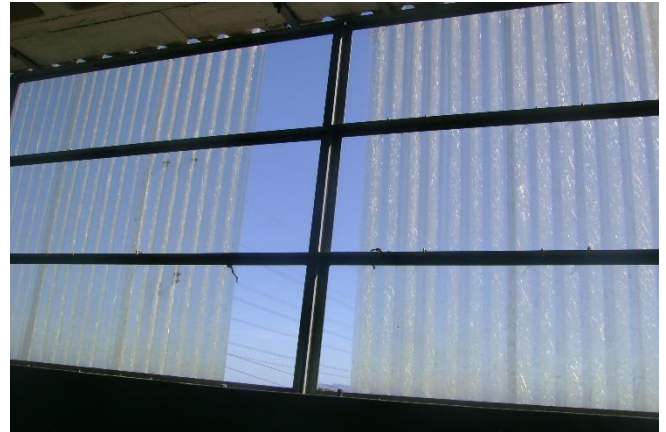
Figure 35: broken windows in station
