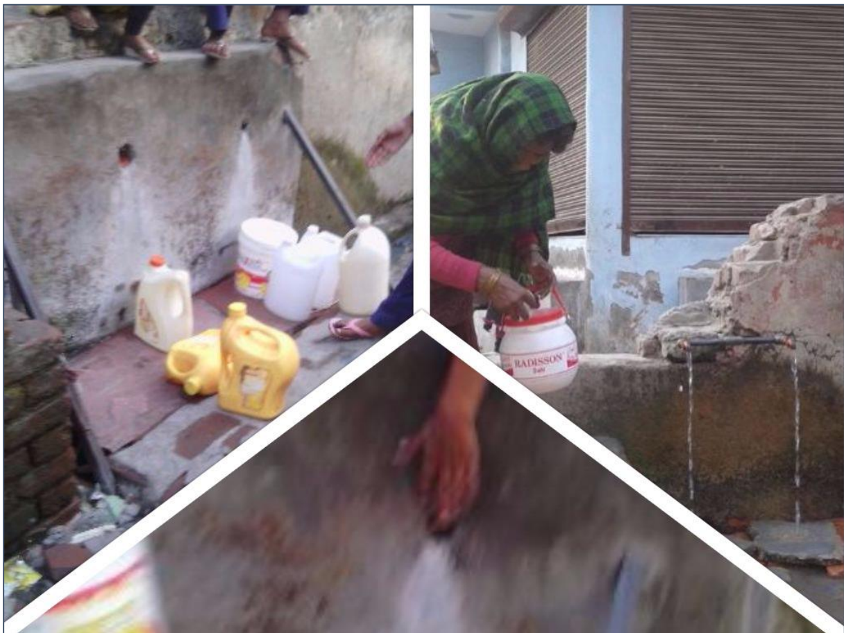
Figure 26 Broken taps, water leakages are common in the area -All participants (Group discussions)
